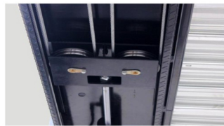
上主平台下滑轮及电缆 Pulley and cable under upper main platform
